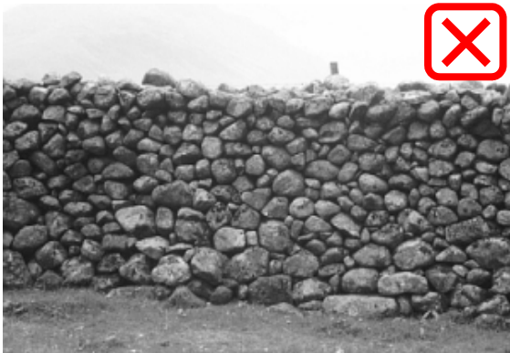
Weak masonry with round shaped stones
