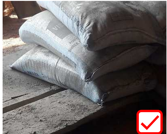
Cement stored above wooden plank
