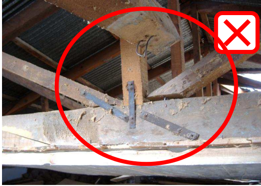
Improper connection of wooden truss
