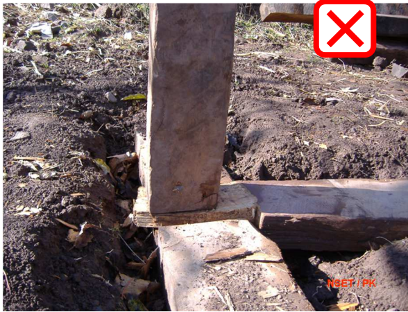
Improper Wooden connection at ground floor level
