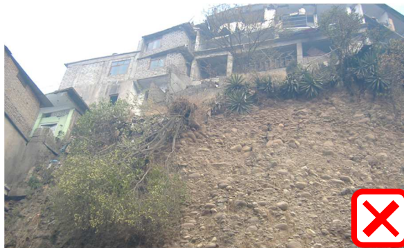
Above land slide prone area
