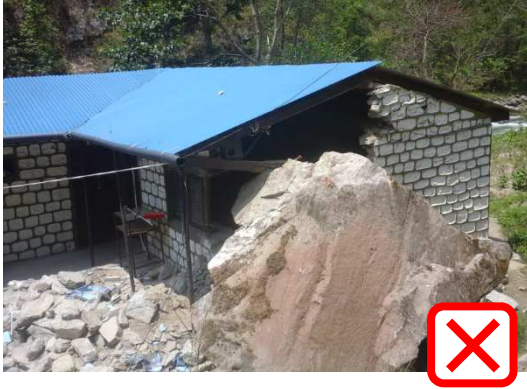
Damage to building due to rockfall
