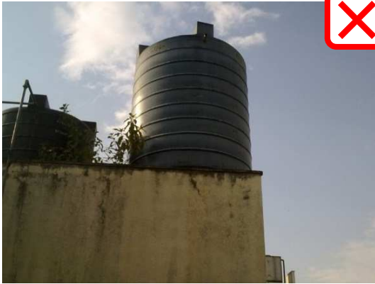
Water tank placed at roof corner without any protection
