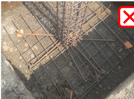
Ends of footing mesh not bent up
