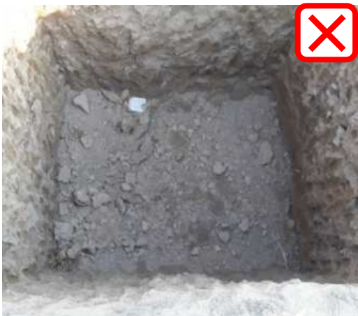
Poorly compacted earth
