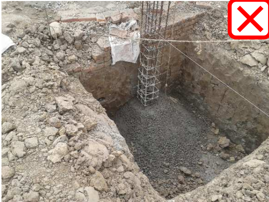
Strap beam not provided for eccentric column
