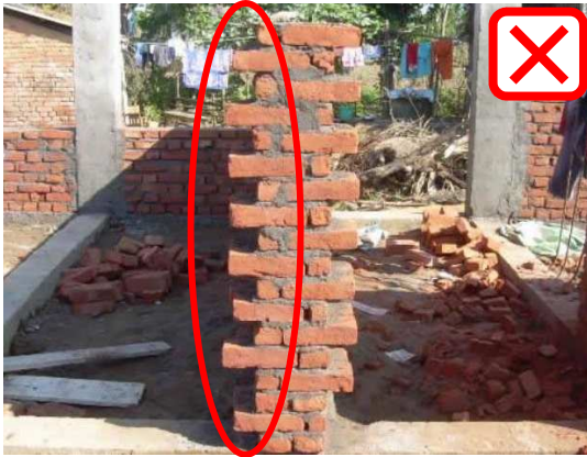
Toothing left for later construction joint
