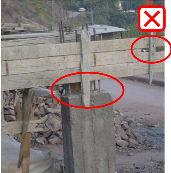
Improper method of formwork
