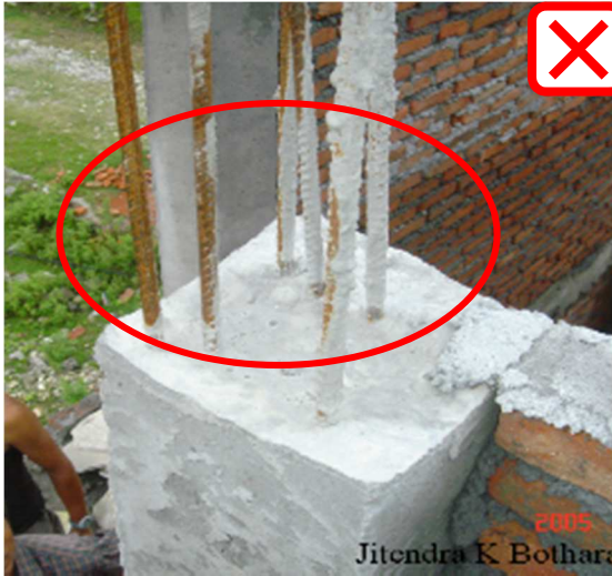
Lack of stirrups above column to hold the reinforcement in position
