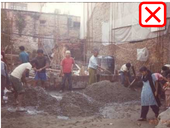
Concrete mixing manually with poor quality
