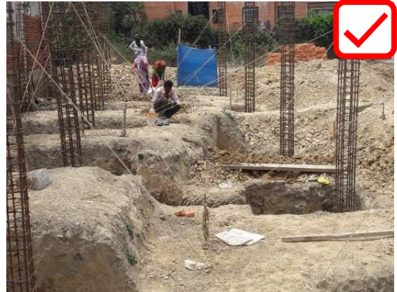
Excavated soil not cleared from site
