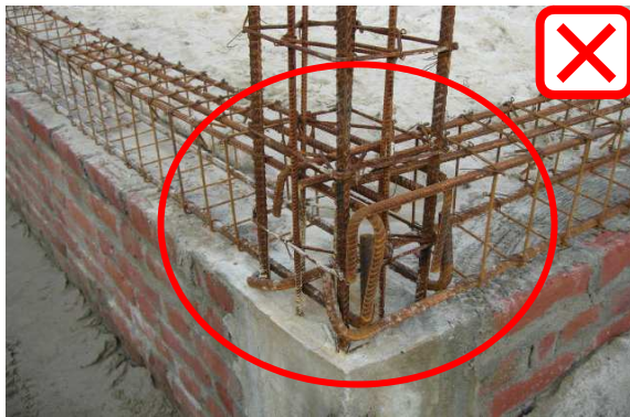
The case where beam reinforcement passing outside of column reinforcement
