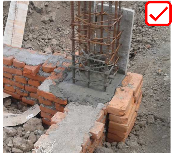
Proper way of using stirrups above casted concrete ( spacing of stirrups shall not be more than 100 mm or as specified in design)
