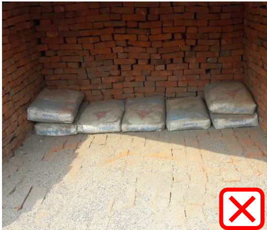
Cement stored in ground above brick soling
